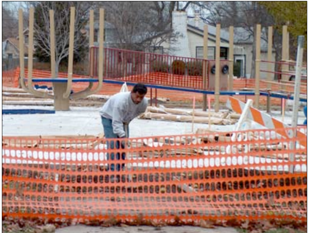
Above, a construction worker prepares the area before the sidewalk is poured that will encircle the new "inclusionary" playground at Summit Park in El Dorado.
