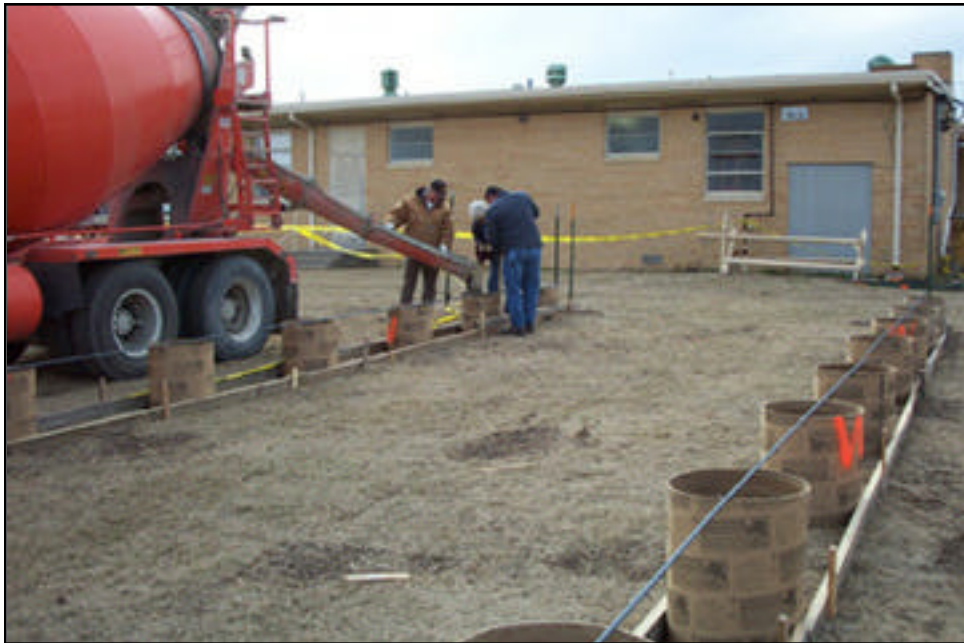
Left to right, Jerry Clark, Greg Buster and Mitch Miller, pour cement in the footings for one of the mobile units which will be moved to the Prospect campus early this spring. (In the background is the northeast corner of Prospect School.) The mobile units will house ACE School which is currently located downtown El Dorado.
